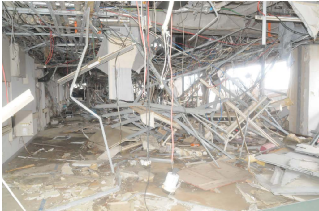
Figure 3: Damages Caused by Tsunami after the Great East Japan Earthquake
